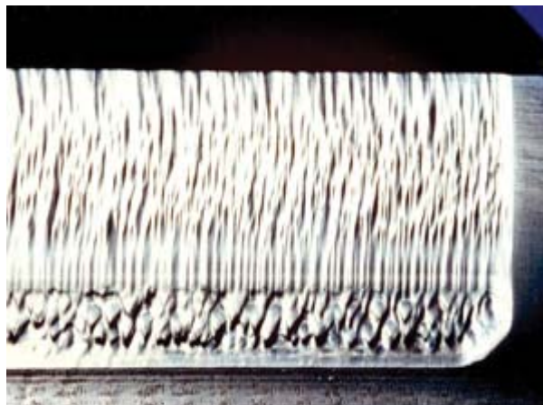
A lubricant contaminated by sand resulted in abrasion on this spur pinion.
