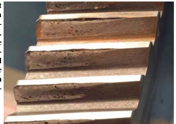
This image shows how severe misalignment can limit the contact area and cause macropitting
